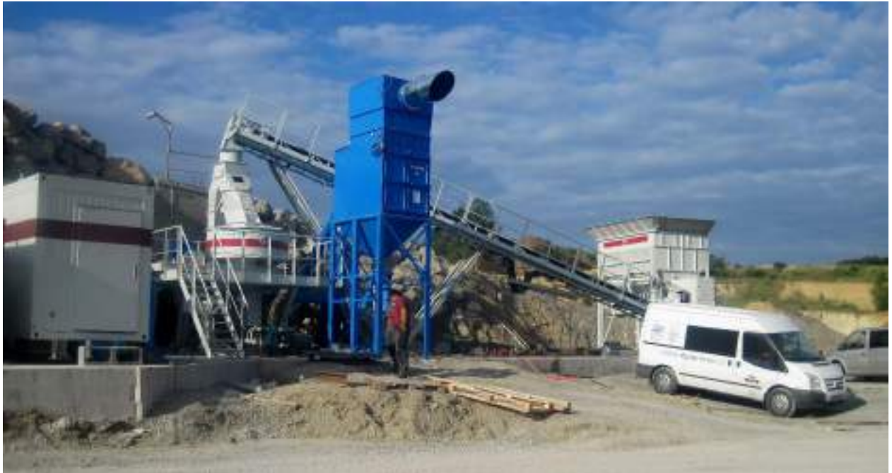
KALCIT s.r.o. Brno – quarry Líšeň (Czech Republic) – limestone processing – VSI crusher VIC 80
