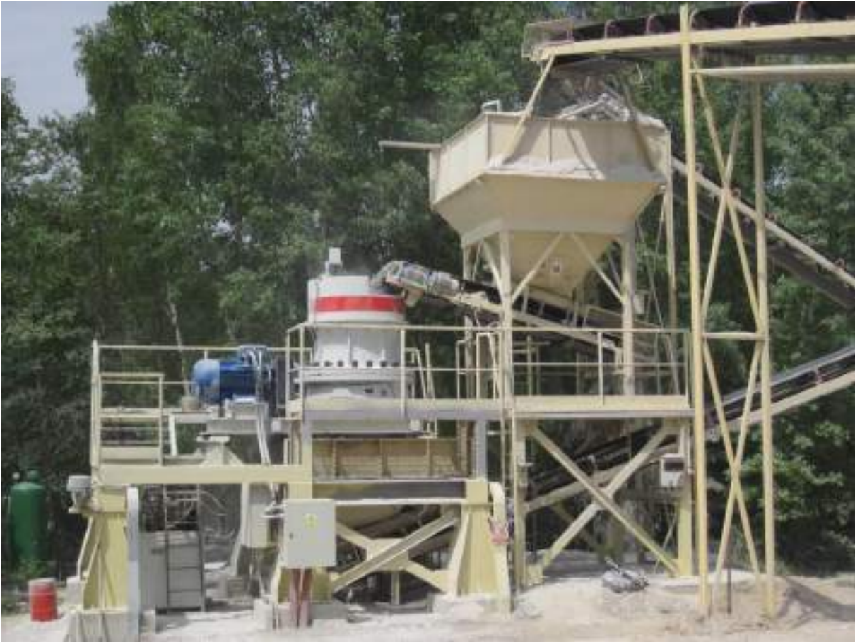
MLADOVICE (Czech Republic) – cone crusher HCU 10/65
