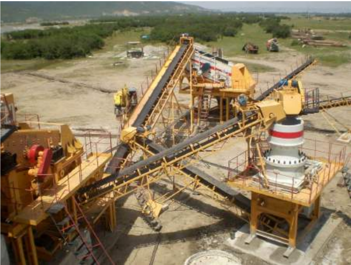
GROZNYJ (Chechnya) – Gravel sand processing plant - HCC 12/65, VTK 200x500/3
