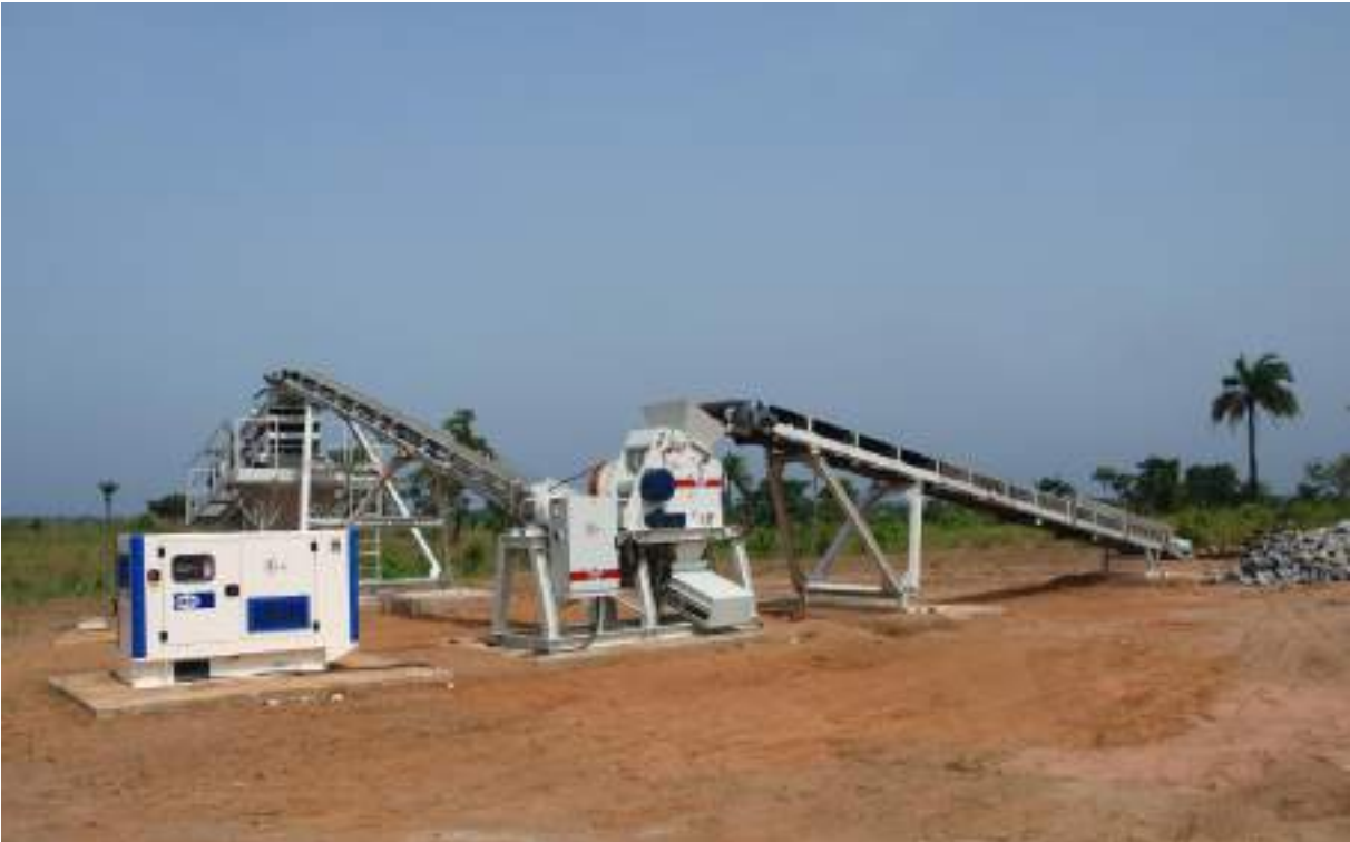
Nigeria – laterite processing plant 25 tph
