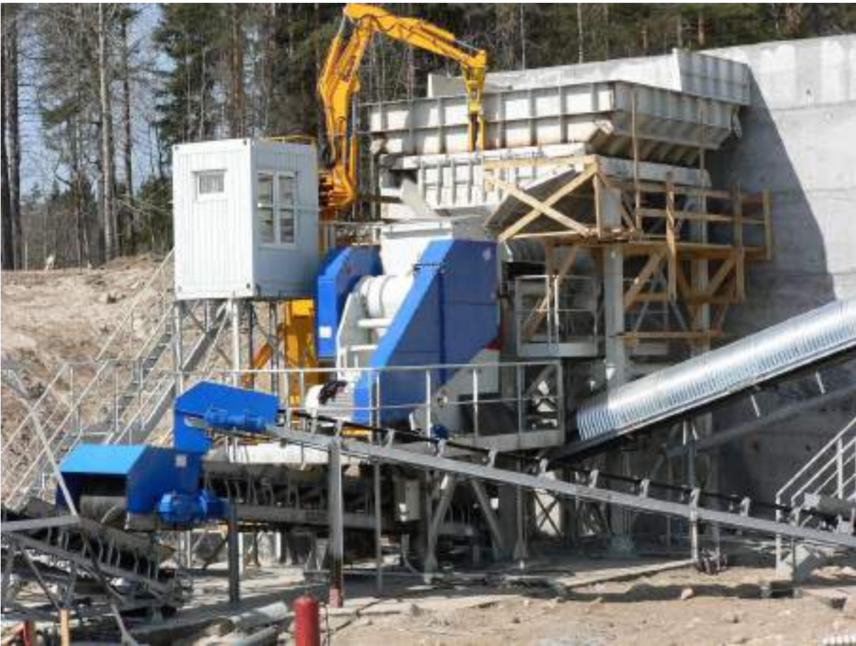
ALCHO (Russia) – Diorite processing plant 200 tph
