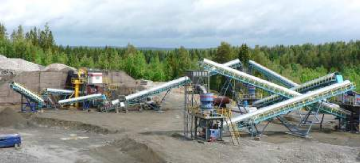
LJASKELJA (Russia) – Granite processing plant 270 tph
