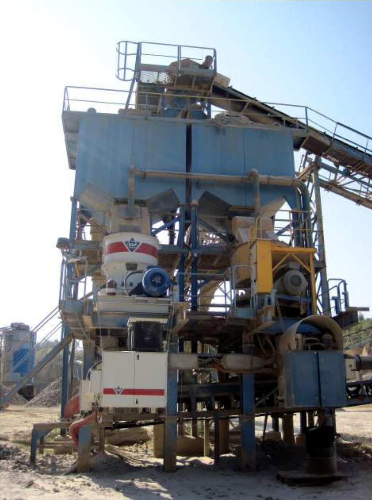
Granita s.r.o. Skuteč – quarry Chvaletice (Czech Republic) – cone crusher HCU 10/90
